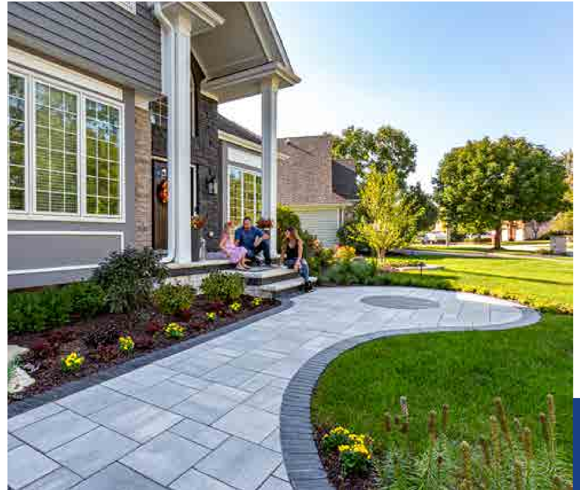
Pavers: Beacon Hill™ Smooth (Granite Fusion) with Cophorne (Basalt) accents Steps: Cophorne (Basalt) accent fascia with LedgeStone™ (Buff) step treads
