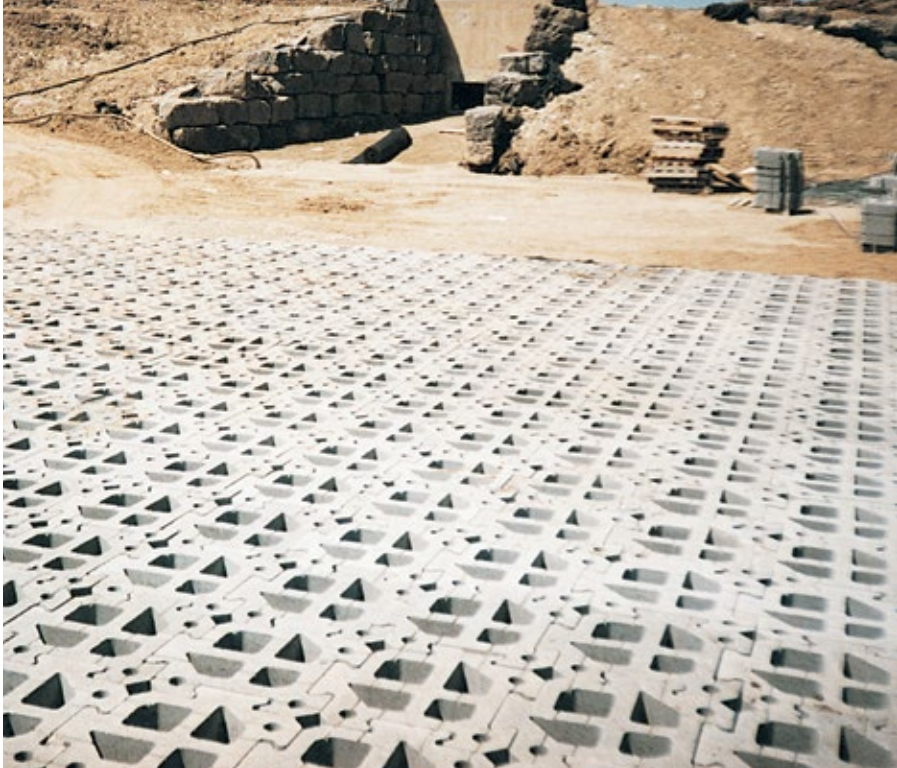
Product: DuraMat Project: Retention Pond
